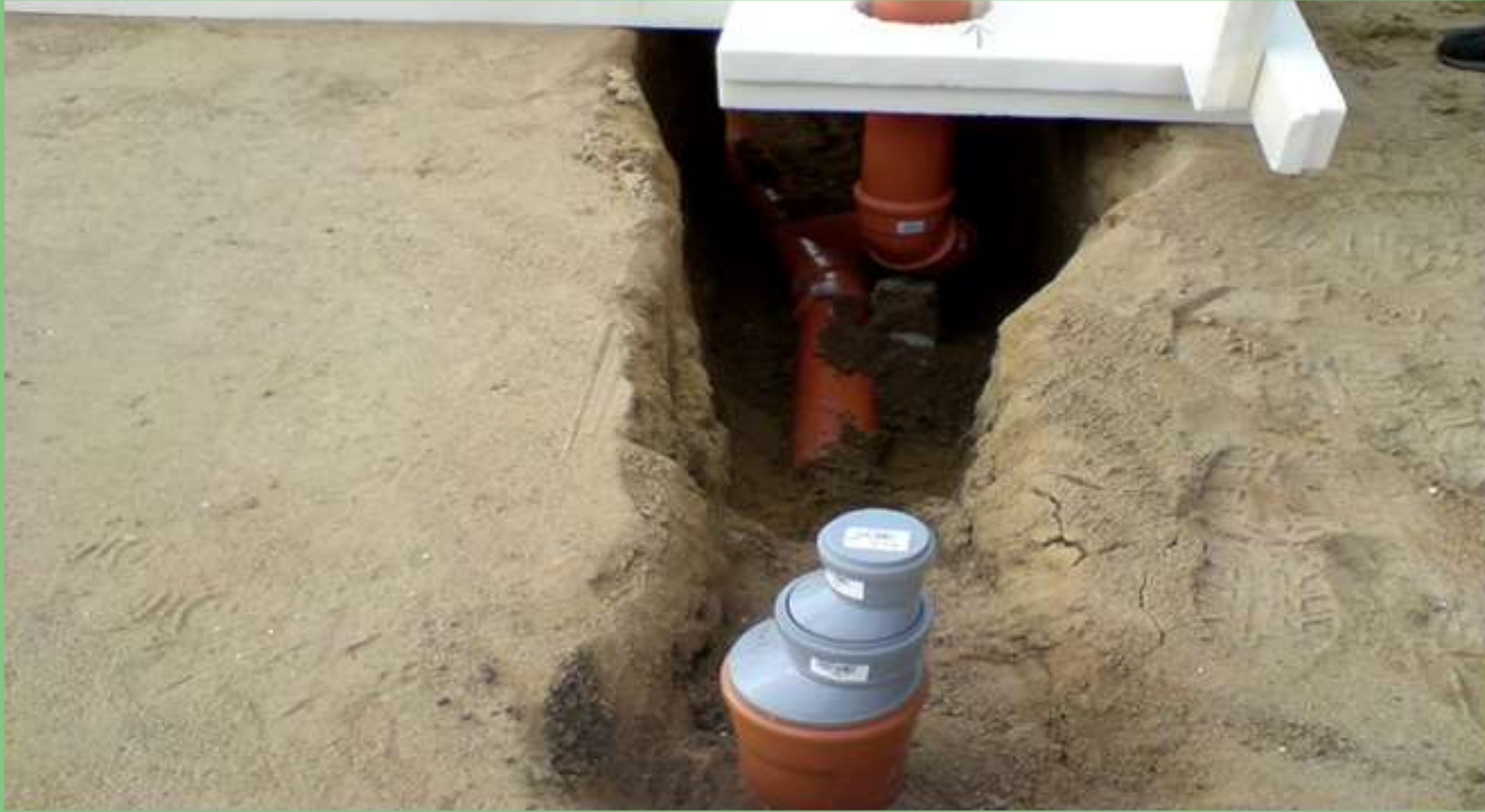
Sewage lines with traps
